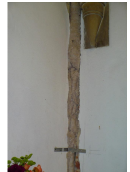
Internal cracks in South wall of the Chancel
